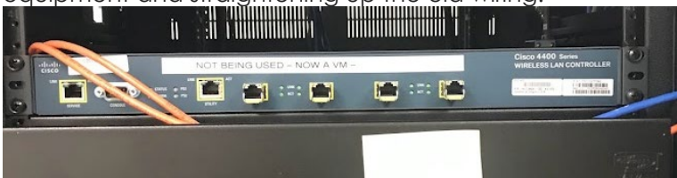
Old Wireless Lan Controller which was previously decommissioned.
