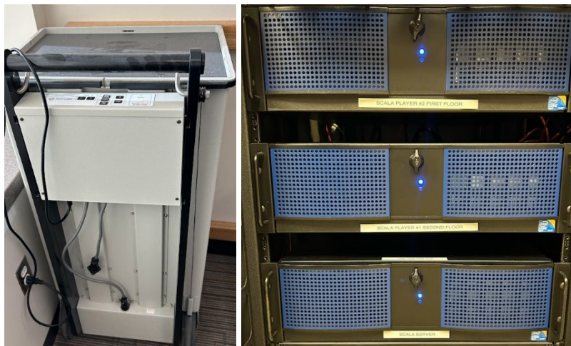
Repaired AST "Brain Box" SCALA server in our server room rack
