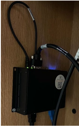
New A/V Transmitter in the Upstairs Meeting Room
